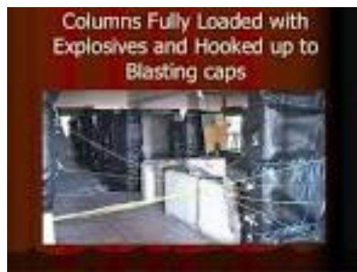
Fig.3.3.Columns fully loaded with explosives and hooked up to blasting caps and fuses.
